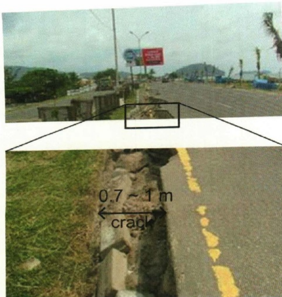
Fig. 4.7 Lateral spreading affecting the Seafront road (Jalan Samaudra) in Padang
