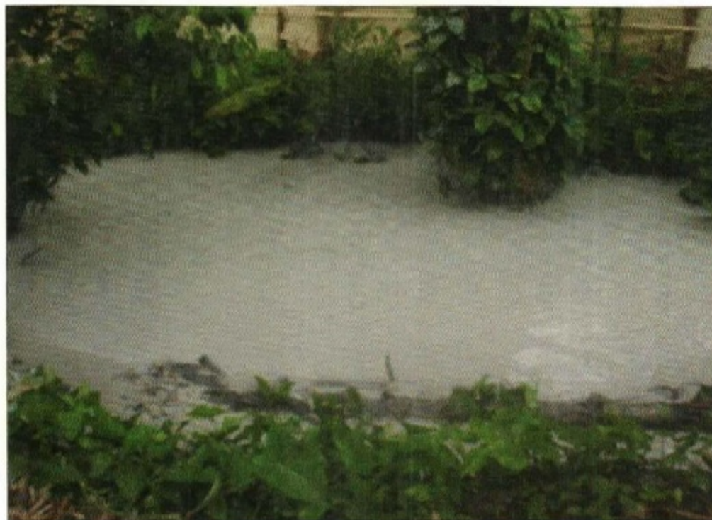
Fig. 4.11 Sand boiling at Kp. Pasir gedc, Sukahening village, Sukahening, Tasikmalaya
