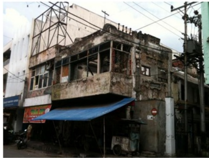
Figure 8 Deterioration of the buildings
