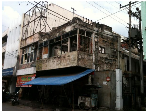
Figure 8 Deterioration of the buildings
