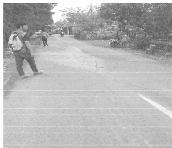
Fig. 4. Land slide under the road
