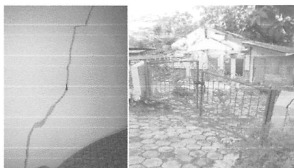
Fig. 3. Houses that are cracked and impacts close to the wells.
