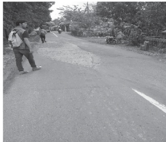
Fig. 4. Land slide under the road
