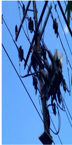
Gambar 2.9 Load Break Switch [27] .
