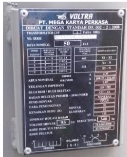
Gambar 2.5 Name Plate Trafo
