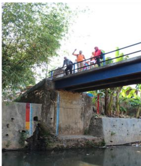
Figure 6. The River Water Level Board TMA at Tikung Bridge Wonosari
