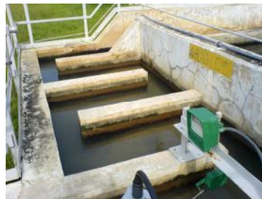
Chlorine Contact Tank
