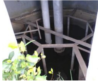
Sludge Collecting Tank
