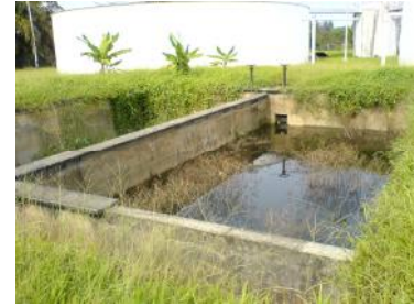
Sludge Drying Bed
